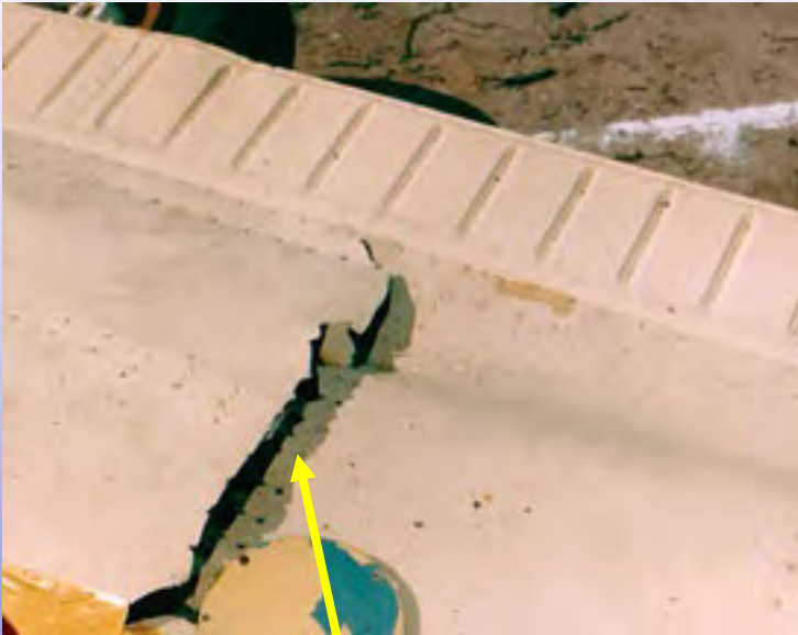
Rivet Line Skin Failure
