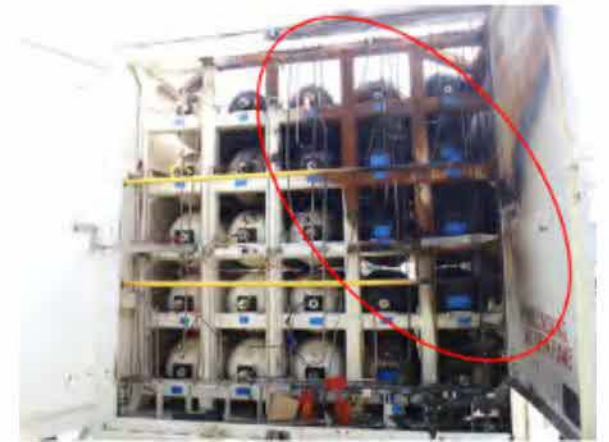
Figure 50. The circled area above shows the sections of the tube trailer module that suffered the greatest thermal damage in the Air Products and Chemicals Inc. truck-tractor fire.
