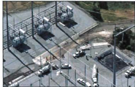
Figure 1 – (U) Damaged transformer at Metcalf Substation
